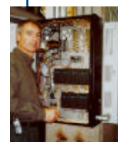
George McFee inspects the Continuum hardware one level below the Gampel basketball court.
