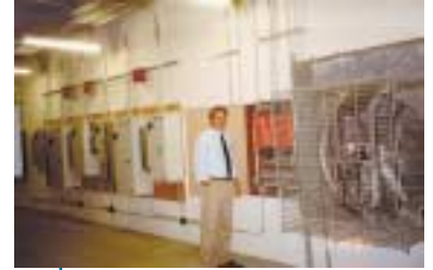
Dean Head, Moffitt's Director of Facilities, inspects some Andover controllers
