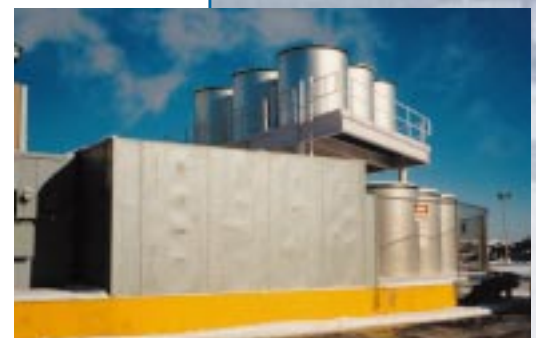
A District 214 ice storage system
