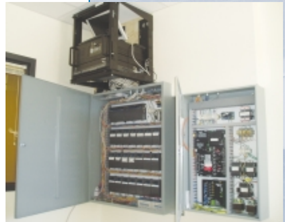
Integrated CCTV, access control, and HVAC system equipment
